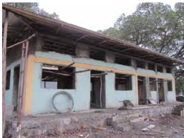
Tuberculosis Unit renovations at Gondar University Hospital, Ethiopia to make improvements in the TB-IC.
