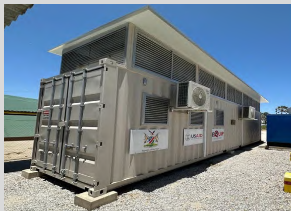
PSA plant installed at Onandjokwe intermediate Referral Hospital and managed by AGS. Photo credit: AGS and MHSS Onandjokwe Intermediate Referral Hospital
